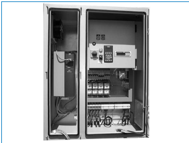
Control Panel with Variable Frequency Drive
