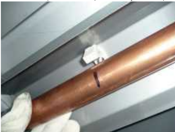
Alignment of waterfeed pipe
